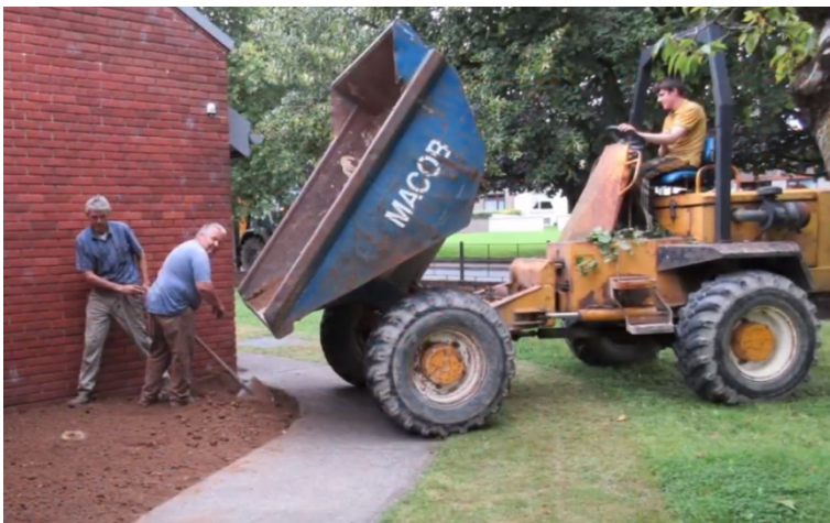
After calculating how much top soil was needed, the soil was delivered and spread across the site.
